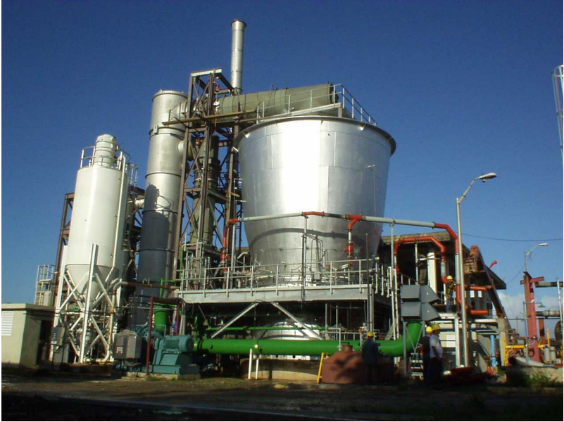
Incinerator for Puerto Rico (4.68m diameter)
