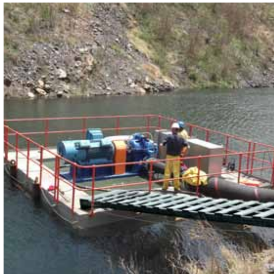
450kw pump set on an 18 ton pontoon
